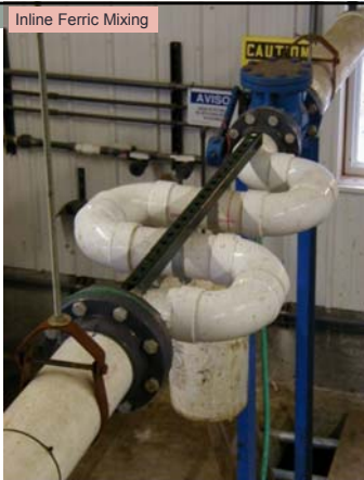
Inline Ferric Mixing
