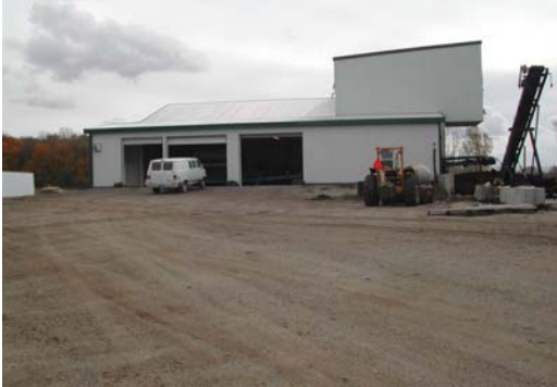
Chemical Phosphorus Separation System
