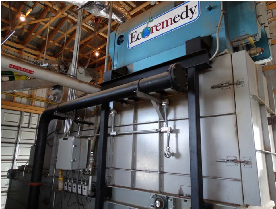
Figure 2. The gasifier is the gray colored device and the boiler is the blue colored equipment at the top. The litter flows through the unit from left to right.
