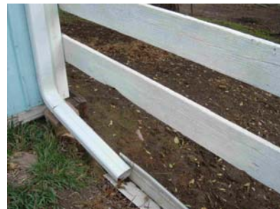
Figure 2. Shed with gutter drainage system. Gutters prevent roof drainage from entering lot.
