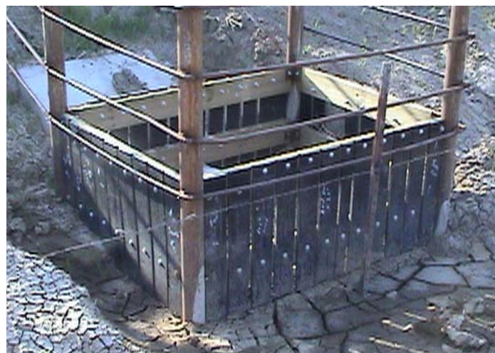
Figure 3. An outlet from a settling basin should screen debris and limit solids' movement into a VTA.
