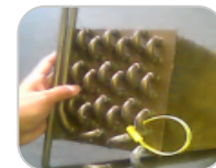
Protective Coating on Evaporator Coils
